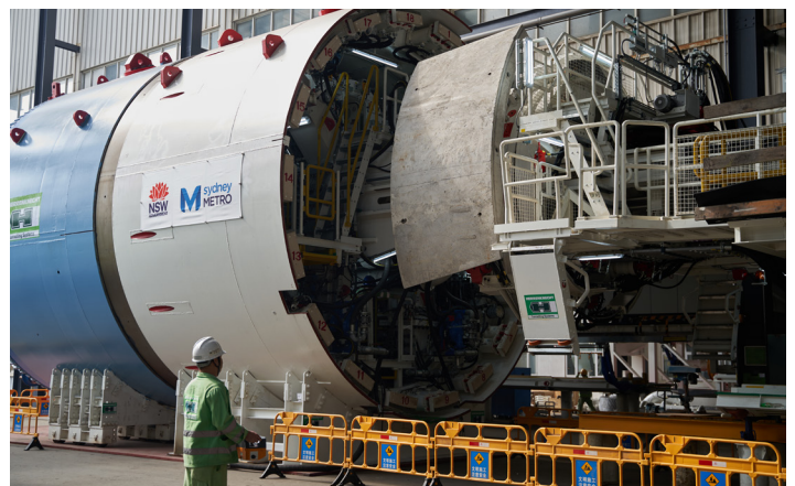
Testing the TBM – you can see one of the concrete segments that will be used to line the tunnels.
